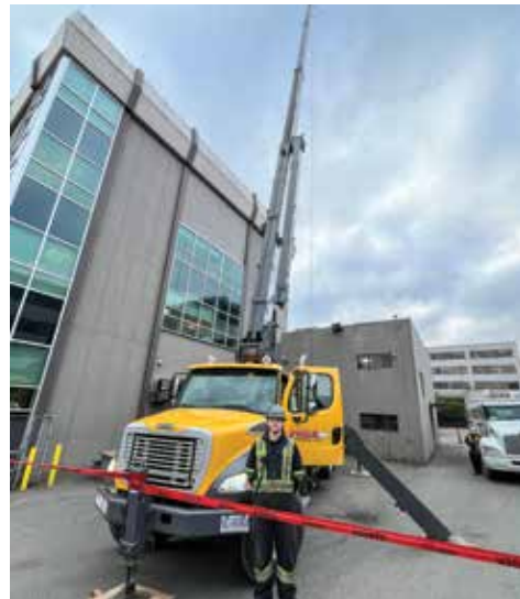
Eagle Crane member North Cummins lifting the new HVAC into place at the Local 115 Burnaby Hall.
