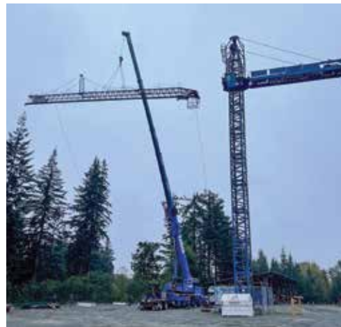
IUOE members working on disassembling the Linden tower crane with the help of mobile crane operator Sean Allemang from Kansen Crane Service.
