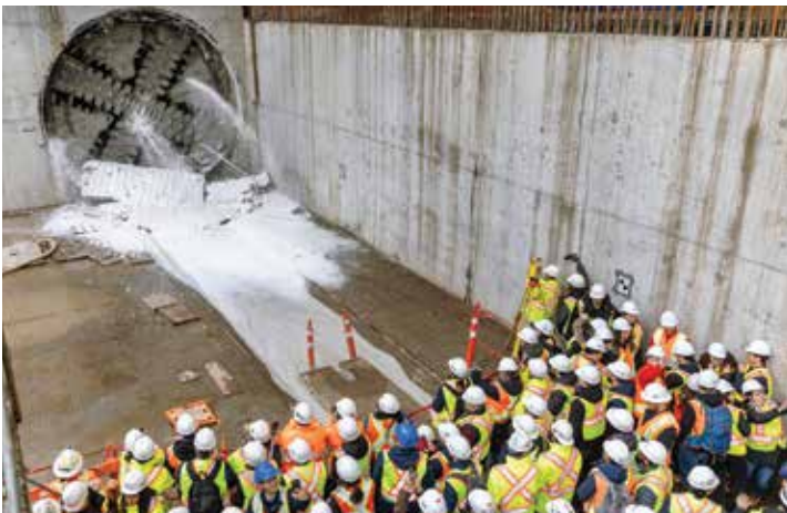
Tunnel boring machine "Elsie" on the Broadway Subway Project, breaking through at the future South Granville Station on February 8, 2024.
