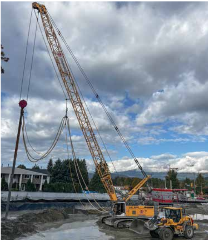
Members working for Menard Canada building stone columns at Port Moody Middle School.
