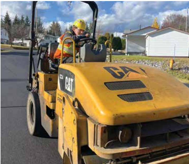
Member Wayne Lussier of Lafarge finishing up a paving job in Prince George.
