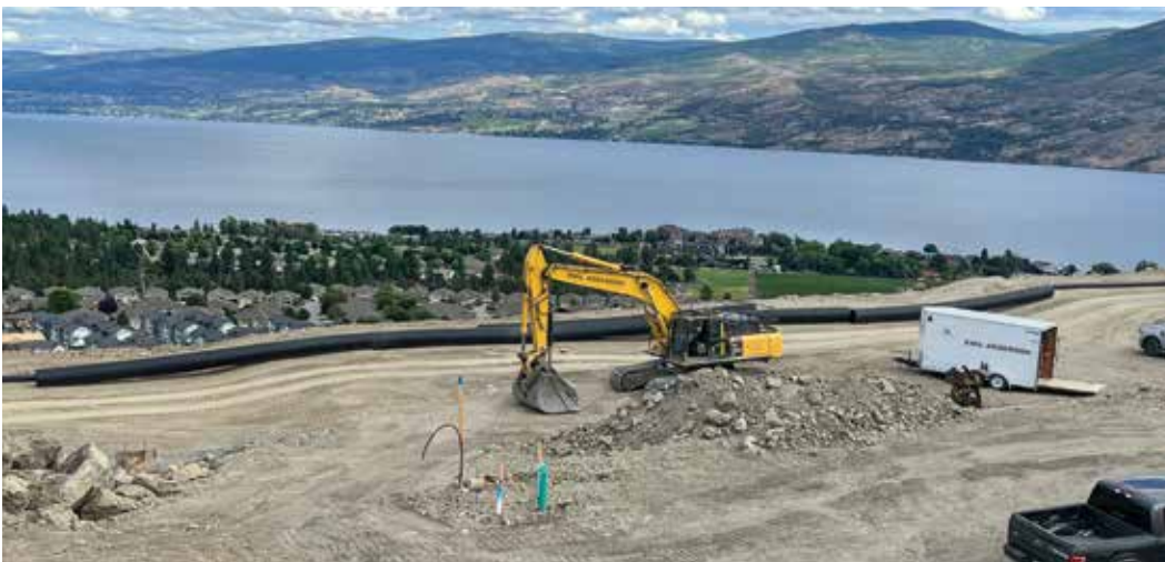
Brother Shawn Irwin working for Emil Anderson Construction at their Shorerise Project in West Kelowna.
