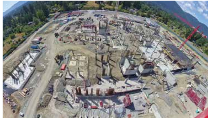
The view from the tower crane at the Cowichan District Hospital Replacement Project.
