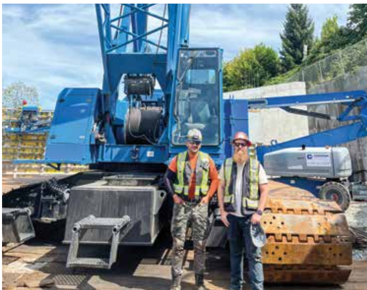
Crane Operators working at the Second Narrows Water Tunnel South Side. L-R: Frank Apel and Warren Torris.
