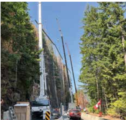
Highway 4 forest fire site; four cranes holding up metal nets preventing debris left from the forest fire from falling on the road potentially closing the vital highway to the west coast once again. Cranes are crewed 24/7.
