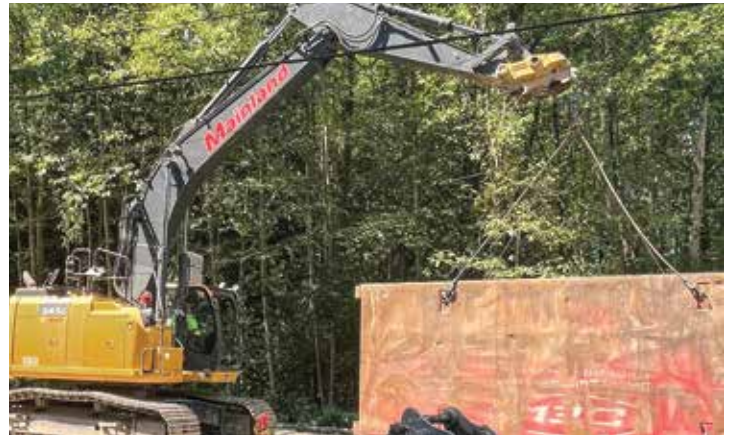
Brian Hynes from Mainland Infrastructure Canada placing a trench box on a project in Langley.
