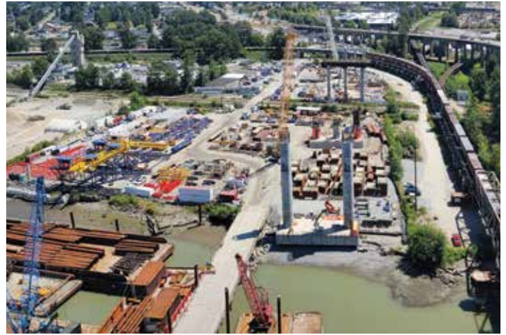
Pattullo Bridge Replacement Project: aerial view of the Surrey approach south. Image courtesy of the B.C. Ministry of Transportation and Infrastructure
