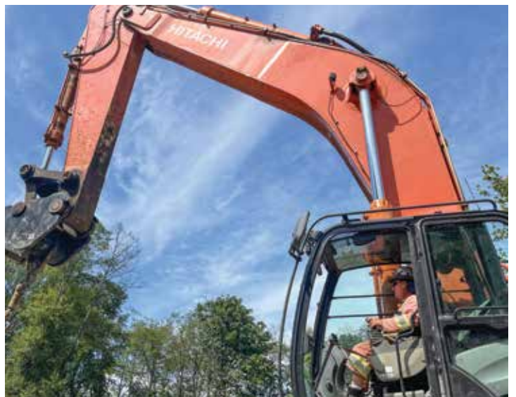
Heavy Equipment Operator Bryant Wishinski working at the Second Narrows Water Tunnel South Side.
