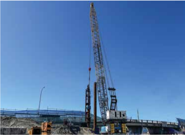
Vancouver Pile Driving working at the Steveston Interchange Project in Richmond, Troy Burstyk at the levers.
