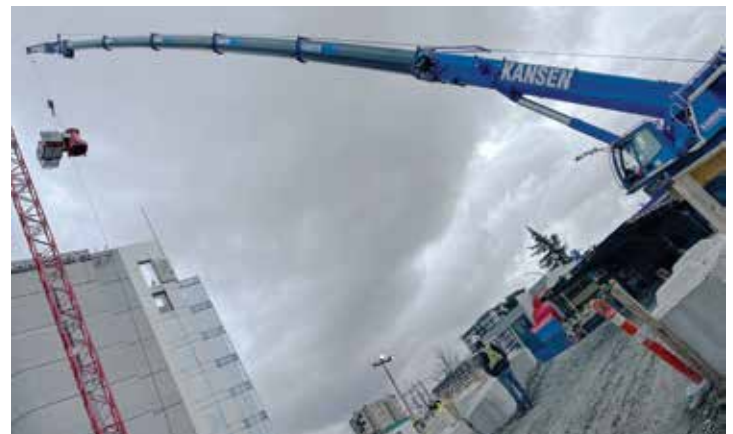
Kansen Crane operator lifting the cab for assembly of the tower crane at the Broadway Subway Expansion Project.
