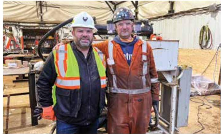
Business Representative Steve Barnicke completes a tour of the Second Narrows Water Supply Tunnel construction site with member Derek Eburne.
