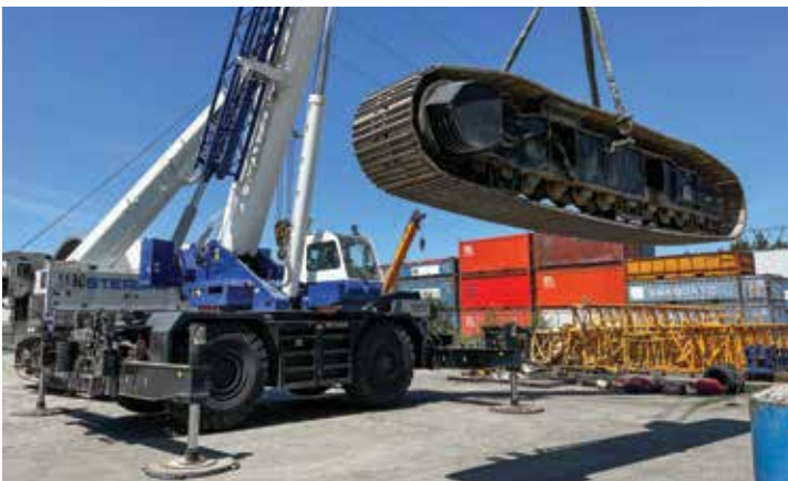
James Kreiser hoisting at the controls at the Sterling Cranes yard in Coquitlam.
