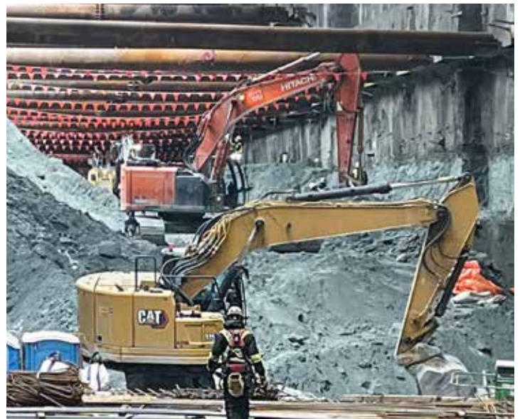
Excavation and shoring crews on tight timelines at the Mount Pleasant location of the Broadway Subway Expansion Project.
