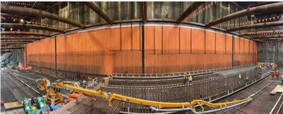
Gastaldo Concrete Ltd. pumping at the City Hall SkyTrain Station Foundation and Tunnel Boring Machine Base.
