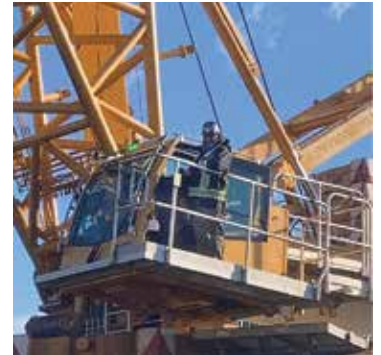
Lonnie Schmidt with apprentice David Lavigne at the controls with LNG Canada.
