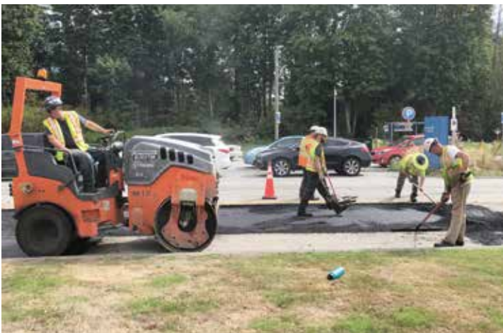
Grandview Blacktop crew working outside of Surrey Memorial Hospital. Luigi (Lui) Tempesta on roller.
