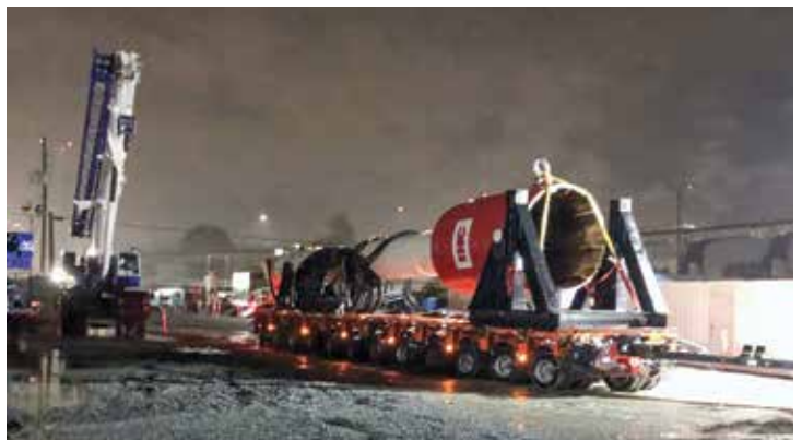
A 66 foot long IHC S800 Hydraulic Hammer weighing 273,000 lbs is delivered to the Pattullo Bridge Project.
