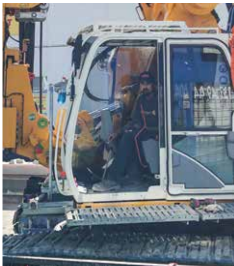
Justin Cusson on a Bauer BG 30 Rotary Drill Rig on the Broadway Subway Project.
