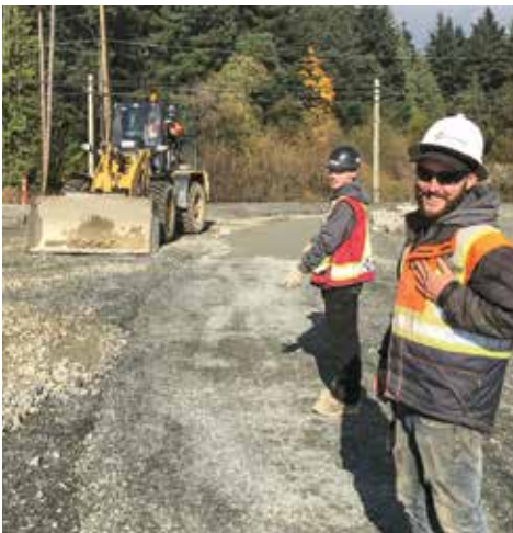
Bailey Busnarda (operating a 918 Wheel Loader) working with Jarud Nicholls and Chris Turner at Hazelwood Construction.
