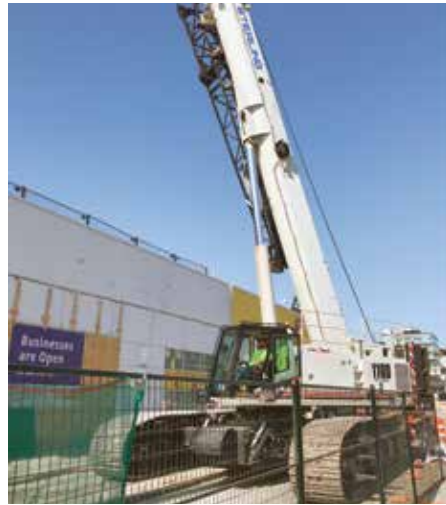
Shop Steward Ken Doan working for BC Infrastructure Benefits at the Broadway Subway Project Site.
