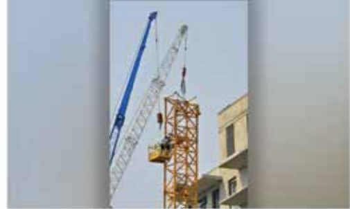
Workers help prepare the upper section of Lethbrun tower crane for removal after its July 12 collapse at a 25-story British Columbia condo project, in which four contractor workers and engineer in adjacent building were killed. PHOTO: Desmond Murray/The Canadian Press via AP
