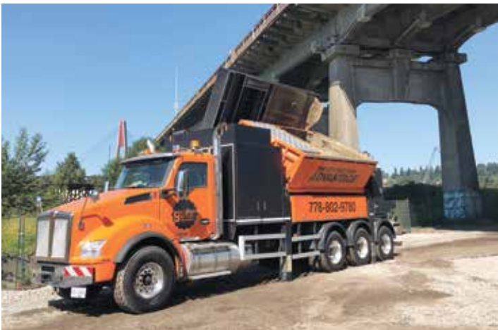
BCIB operator Philip Neufeld working for Gear Equipment at the Pattullo Bridge Replacement Project site.
