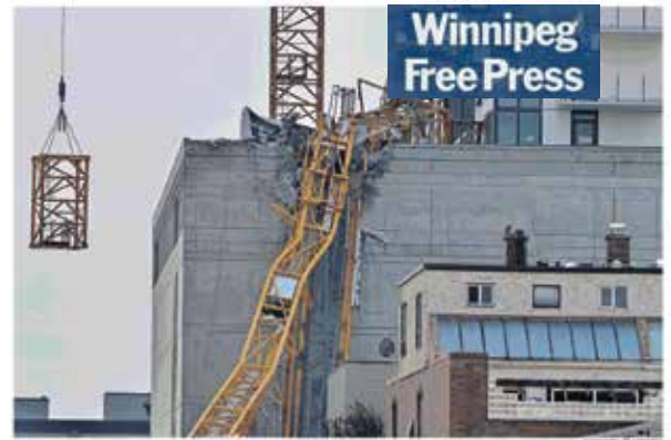
A section left of the vertical column of a construction crane is suspended by the weight of the other tower between B.C., on Wednesday.
