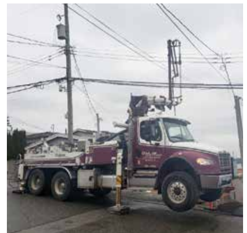
Jesse Tober with Rempel Bros. Concrete navigating wires on a 28 meter Alliance Z boom concrete pump.
