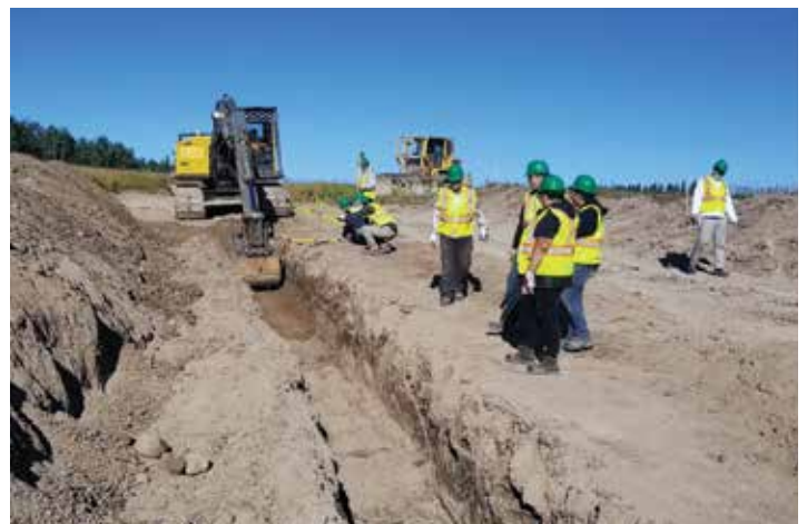
Entry Level Pipeline training for local Indigenous people to work on the Coastal GasLink Pipeline.
