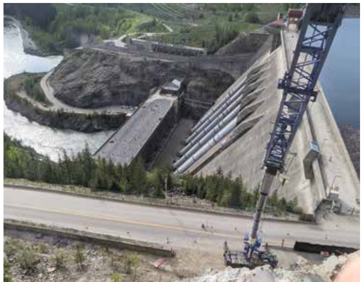
BC Hydro slope stabilization work at Revelstoke dam. Bob Warren operating a Tadano GR-1600XL (160 ton rough terrain crane) with 187 feet main boom plus 59 feet of jib while doing rock bolt layout from a man basket.
