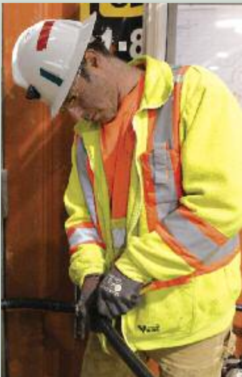
Brian Chaisson, a member of the Electrical Workers Local 230, is replacing the temporary wiring with a more permanent system for the site.
