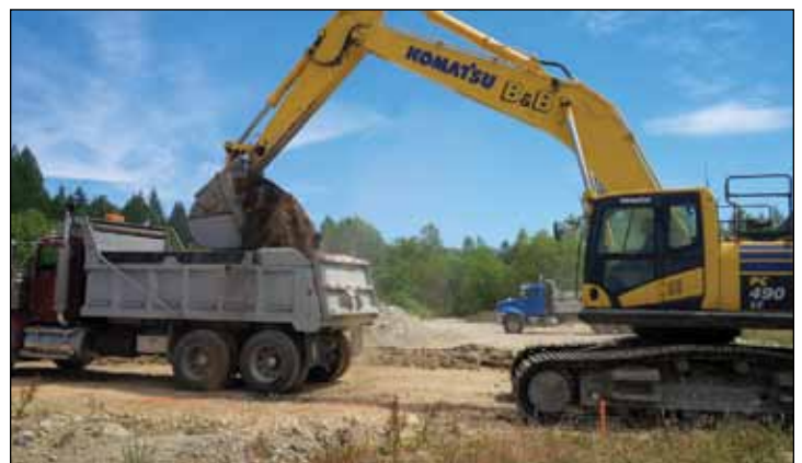
Brother John Young working for B&B Contracting Ltd. at the Grant Hill Subdivision Project in Maple Ridge.
