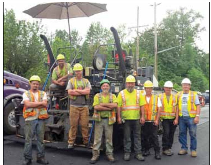
L to R; Brothers Joey Floro, Byron Middleton, JJ Walker, Jack Alves, Joe Leblanc, Steve Rundle, Moises Galvao and Domenico Porchetta with Imperial Paving Limited working on Dewdney Trunk Road in Maple Ridge.
