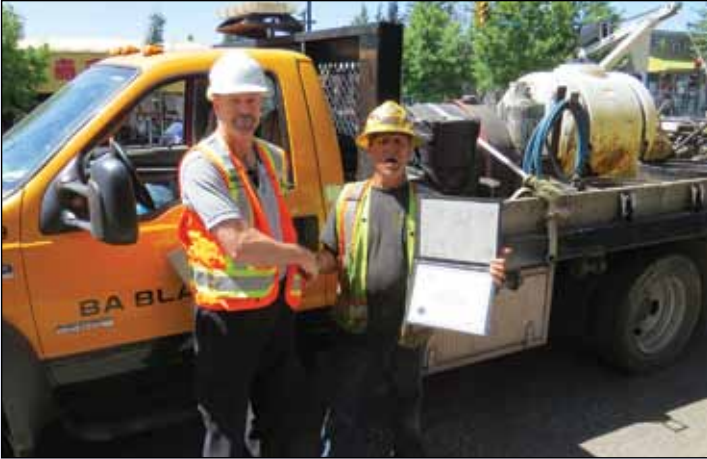
Brother Antonio J. Sousa receives his Asphalt Paving Laydown Certificate of Qualification from Brother Jeff Turner (Training Coordinator) on BA Blacktop's job in North Vancouver on Longsdale and 19th.
