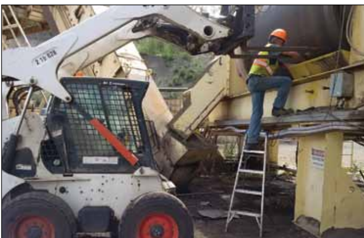
Brothers Chris Kemp and Al Satelmayer replacing a trunnion on the plant at Pittman Ashphalt in Prince George.
