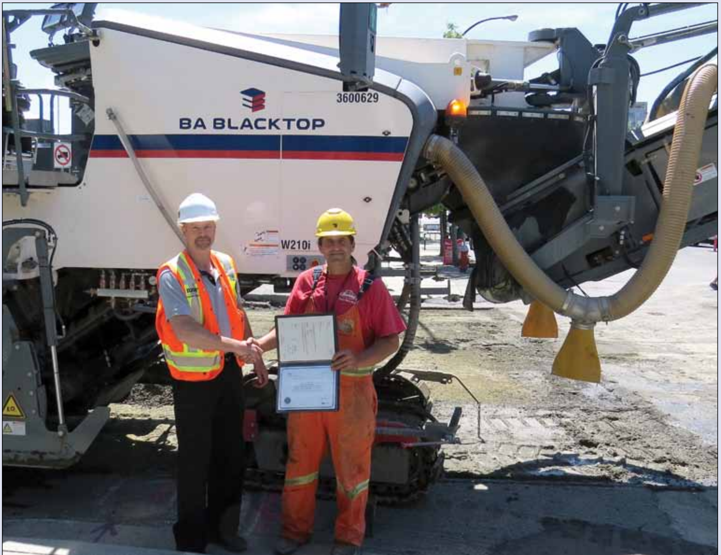
Brother Michael Kullman with B.A. Blacktop Ltd. receives his Asphalt Paving Laydown Certificate from Brother Jeff Turner (Training Coordinator) on Imperial Paving's job at Longsdale and 19th in North Vancouver.
