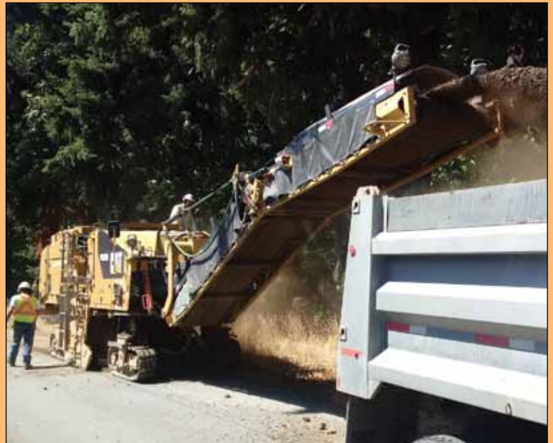
Hub City Milling Division preparing a Port Alberni City municipal utility trench.
