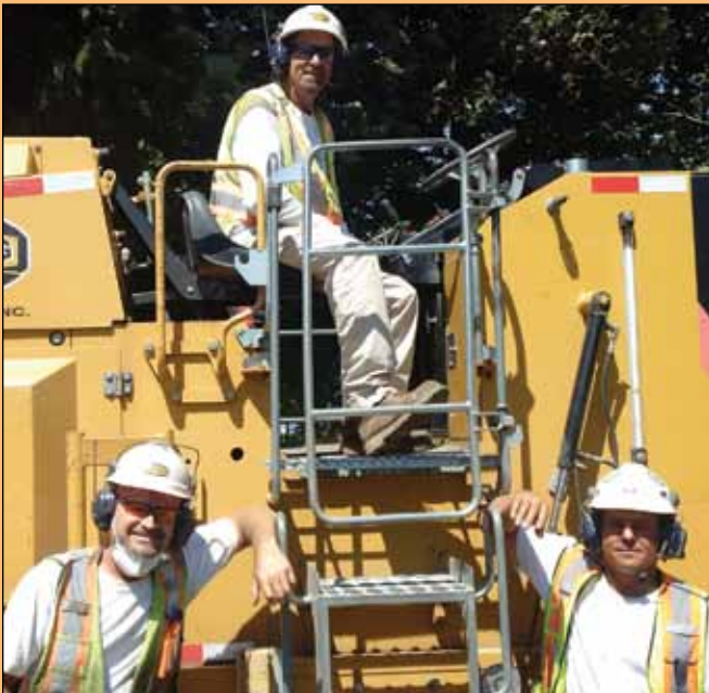
The milling crew of Hub City Milling Division preparing a Port Alberni City municipal utility trench; Brothers Darin Zomar (Foreman), John Olsen and Dave Theriault.
