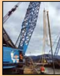
Brother Rob Arnott operating a Manitowoc 4000w for Geopac at the Squamish Terminal dock replacement project.
