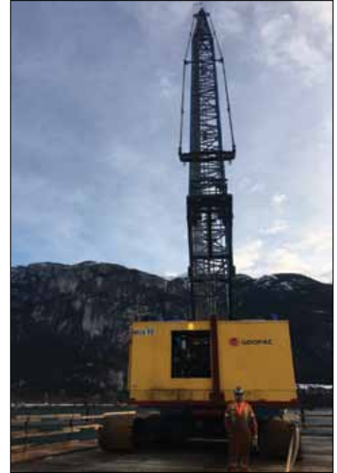
Brother Jason Krickan working for Fraser River Pile at the Squamish Terminal replacement project. He is operating a Manitowoc 4100, building stone columns.
